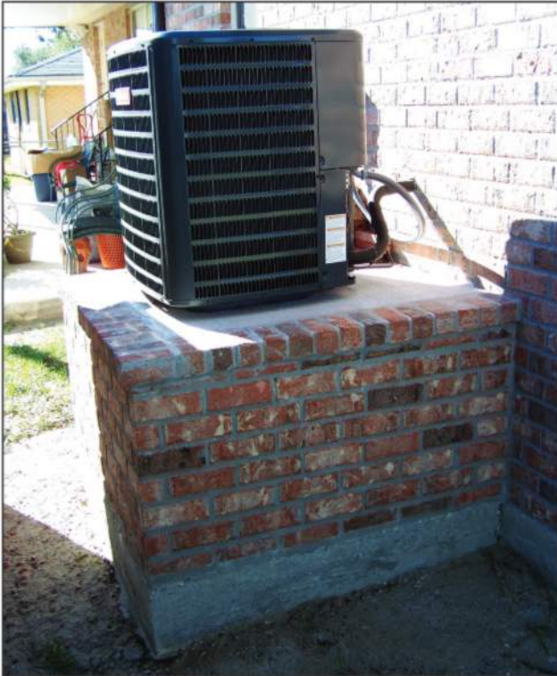
Figure 3-1. Air conditioning compressor elevated on a pedestal.
