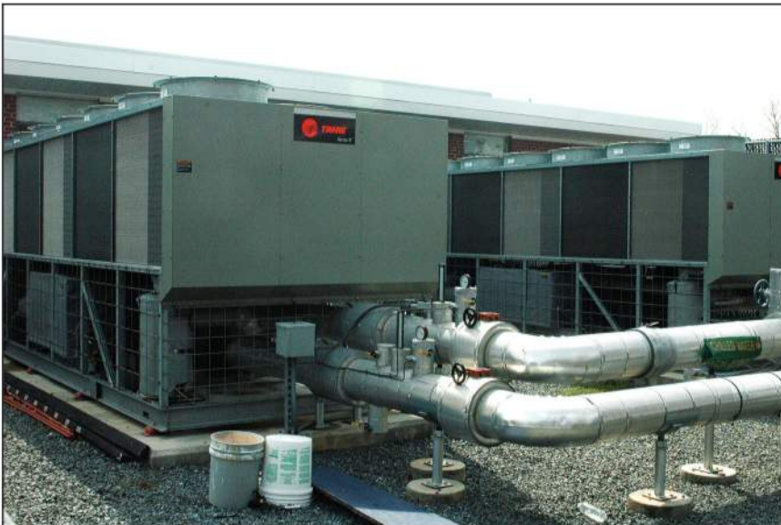
Figure 5-3. Air-Cooled rooftop chiller in Georgetown, Delaware.
