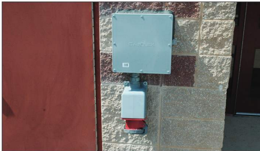
Figure 4-14. Flanged connection (quick connect) for connecting temporary generator (Milford, DE).
