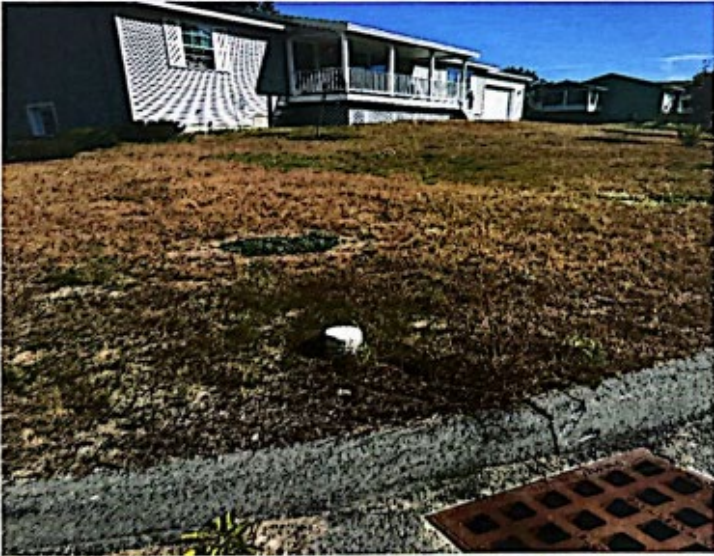
Photograph 16 – Unknown PVC Pipe Within Proposed Town ROW at 29 Homewood Boulevard (Photo Taken by Jaime Wallace, PE Dated September 26, 2023)
