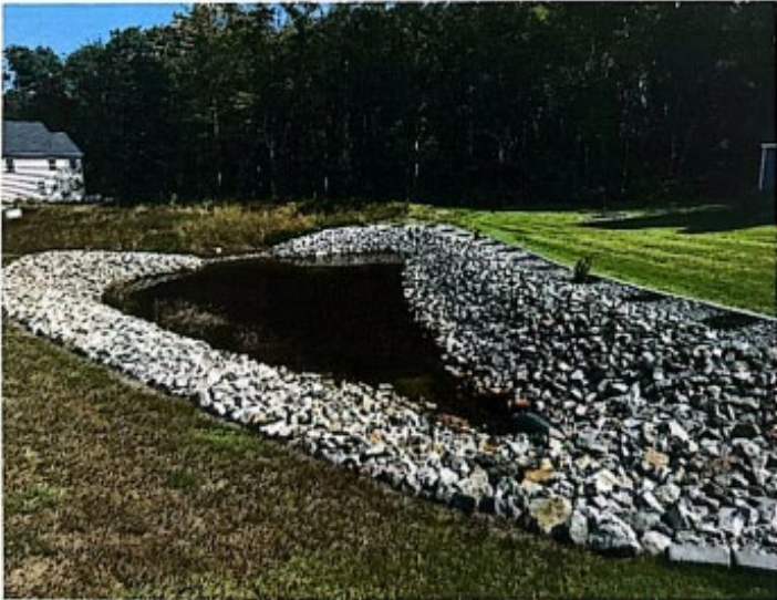
Photograph 12 – Sediment Forebay to Gravel Wetland (Photo Taken by Jaime Wallace, PE Dated September 26, 2023)
