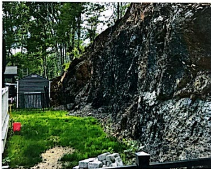
Photograph 2 – Rock Wall Face and Potential Hazard behind 24, 26, 28, and 30 Kapok Street (Photo Taken by Jaime Wallace, PE Dated June 15, 2023)
