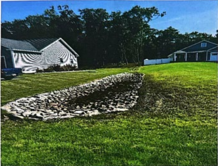
Photograph 11 – Drainage Issues in Swale within Proposed ROW at 17 Kapok Street (Photo Taken by Jaime Wallace, PE Dated September 26, 2023)
