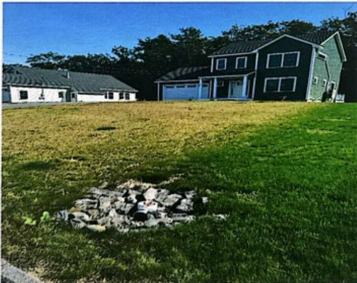
Photograph 10 – Unknown Drainage Structure in Front of 19 Kapok Street (Photo Taken by Jaime Wallace, PE Dated September 26, 2023)
