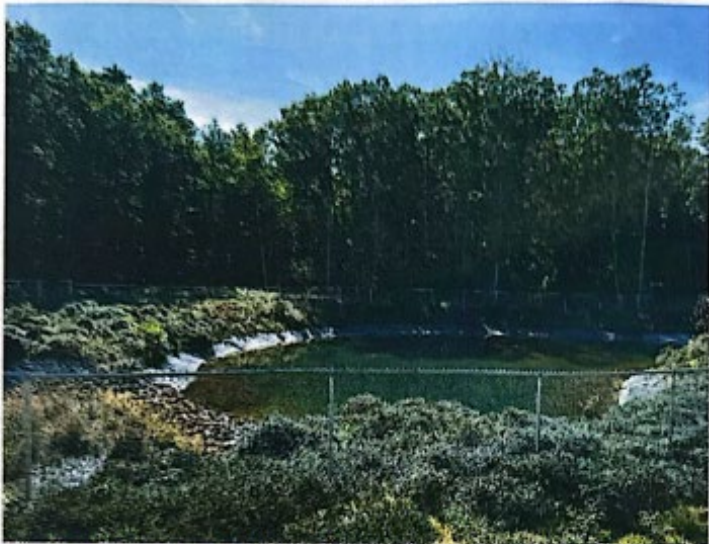
Photograph 5 – Wet Pond with Liner Exposed (Photo Taken by Jaime Wallace, PE Dated September 26, 2023)
