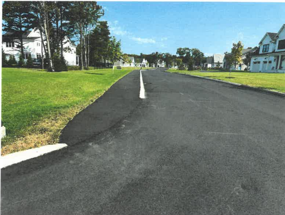
Photo 2: Handicap Detectable Device Needed at End of Summer Long Drive Near Cul-de-Sac (Photo taken by Jaime Wallace, PE dated 9/13/2024).
