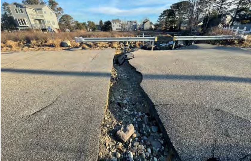
Flood damage on New Salt Road from Winter Storm Elliott in December 2022
