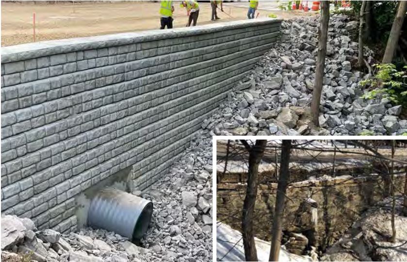
Construction of new retaining wall with previous failing wall and culvert inset.
